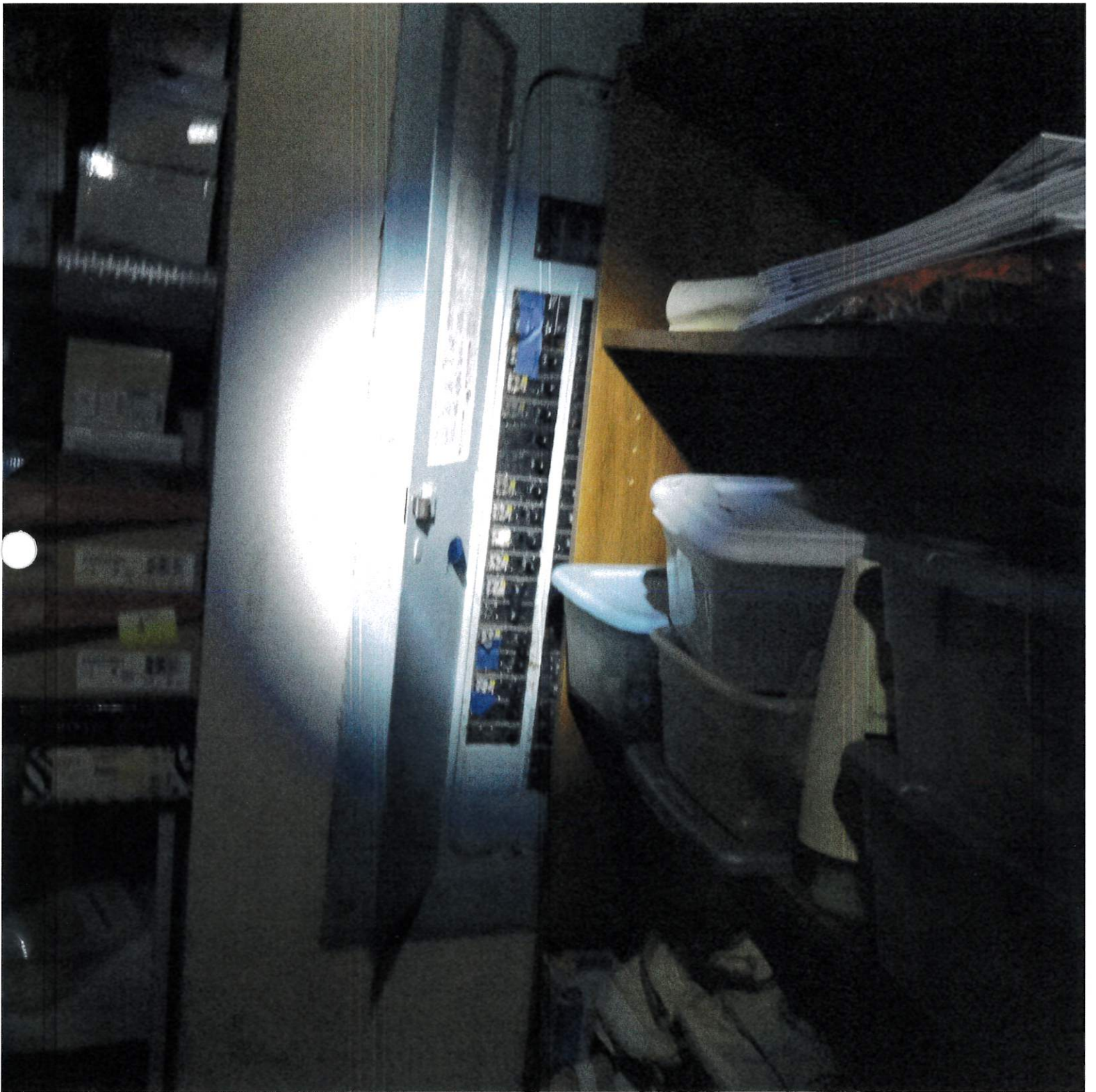
N ACCESSIBLE ELECTRICAL PANEL
