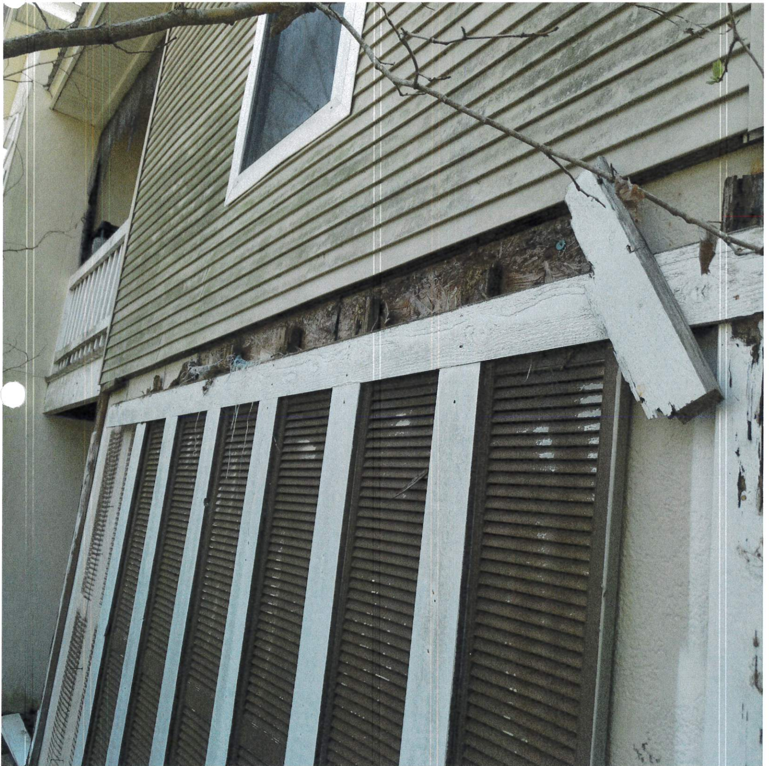
WATER INTRUSION AND TERMITE DAMAGE
