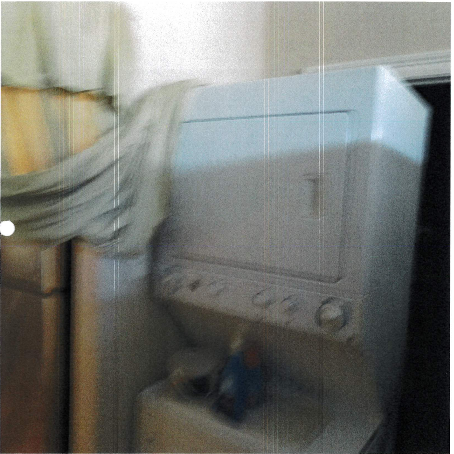
IMPROPERLY VENTED DRYER - VENTED INTO THE ROOM
